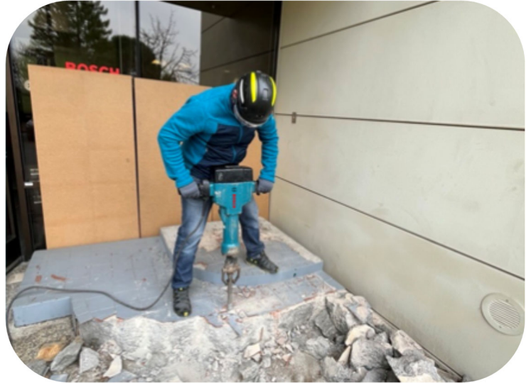
Working #LikeABosch: Can you guess who spent a couple Sunday's helping to clean up the front entrance of Rse 120? Yep, that's new plant manager Christian Foerster safely excavating some old concrete.
